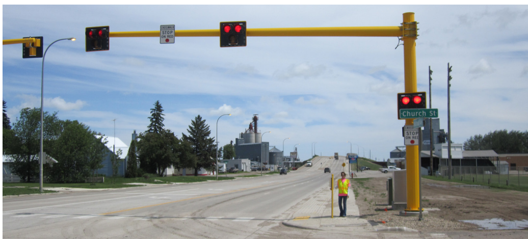
High-Intensity Activated Crosswalk Beacon
